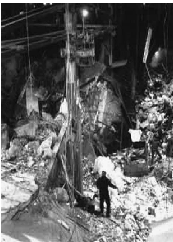
Damage to the garage.
